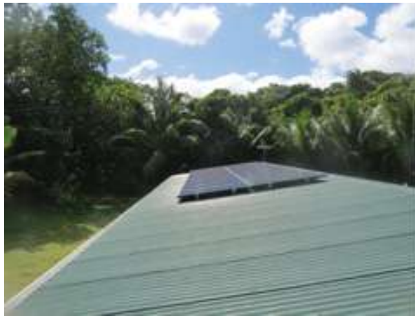
Figure 6: Array on House Roof
