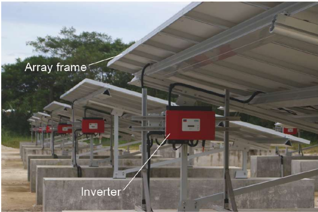
Figure 4: Showing Inverter and Frame
